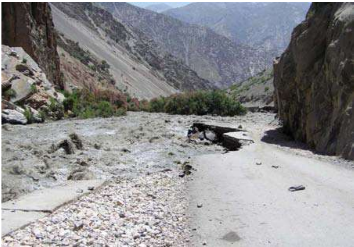
Figure 6: Damage to highway by a flash flood in July 2005 in Garam Chasma, Chitral, Pakistan
